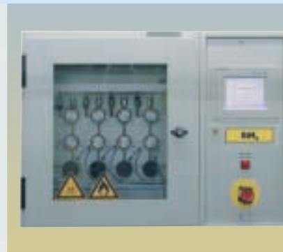
Valve manifold box with S7-200 CPU TP 170A panel
