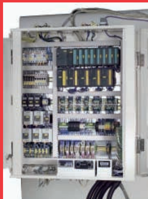
The clean structure of the interior of a typical module control cabinet, with the local control components, including the fail-safe related parts
